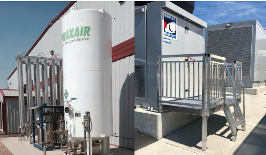
Tank Storage, Generators, Service Yard
