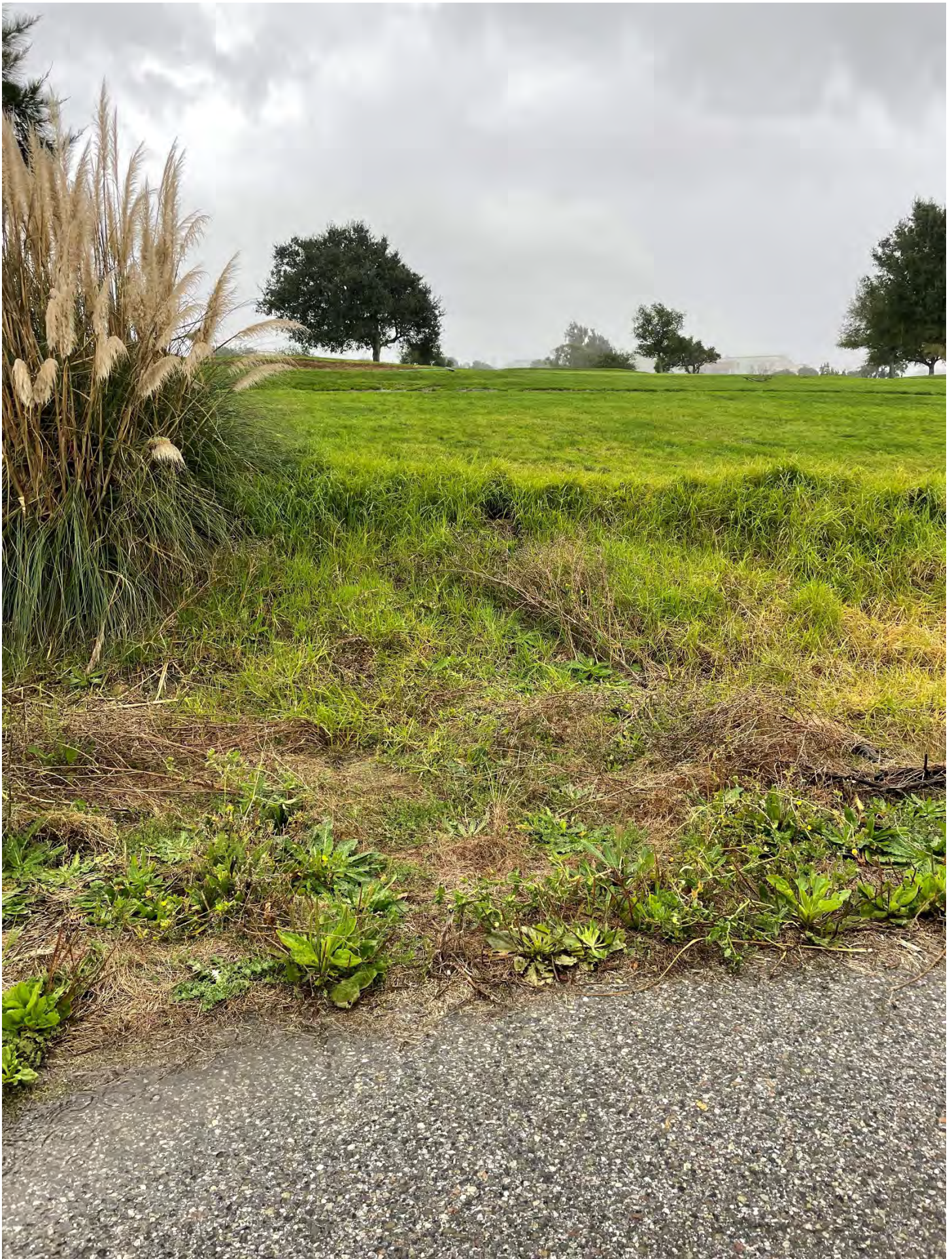
Photo 14: Site 22 - Facing South – Pampas grass and open burrow on north slope. Burrow repaired on February 9, 2024.
